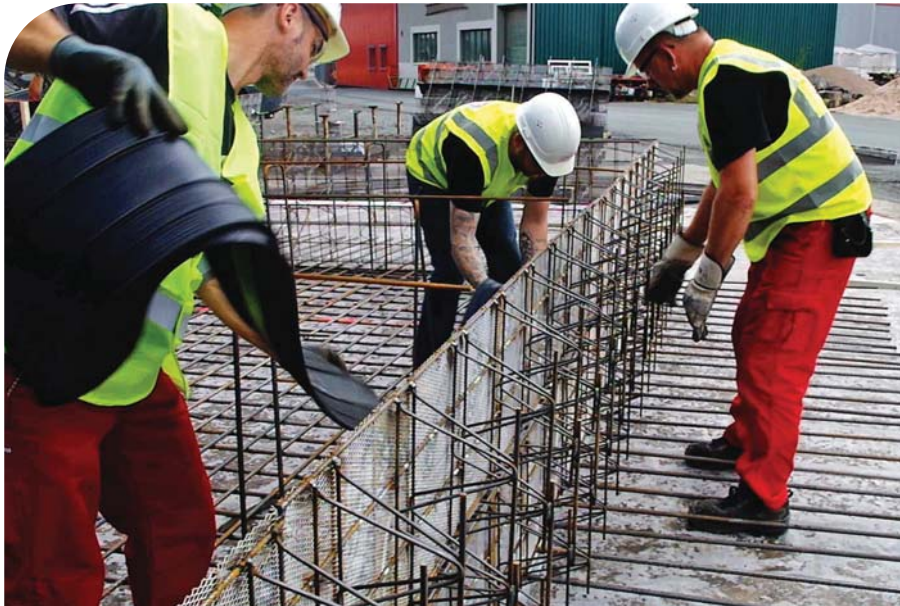
LEFT: Figure 3 – Stremaform enables a sequence of pours and can be supplied including a waterbar cage.
